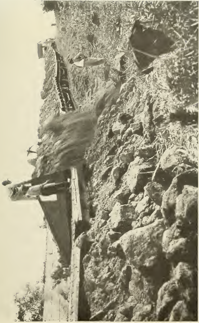
DUMPING "DIRT" FROM CANAL EXCAVATIONS; THE STEEL WEDGE HAULED BY A CHAIN RAPIDLY PUSHES ALL THE DEBRIS ON ONE SIDE.
